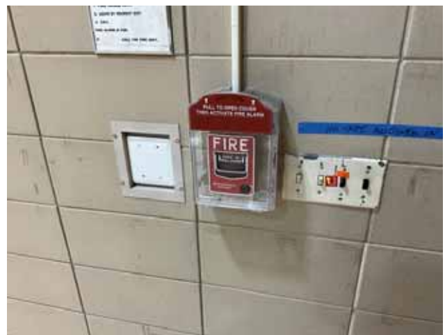
24 - FIRE ALARM DEVICES
