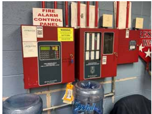
22 - FIRE ALARM PANEL
