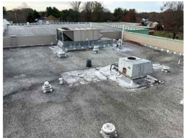
16 - ROOFTOP MECHANICAL EQUIPMENT
