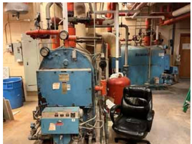
18 - MAIN MECHANICAL ROOM
