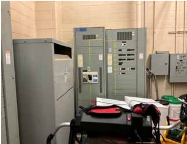
19 - MAIN ELECTRICAL ROOM
